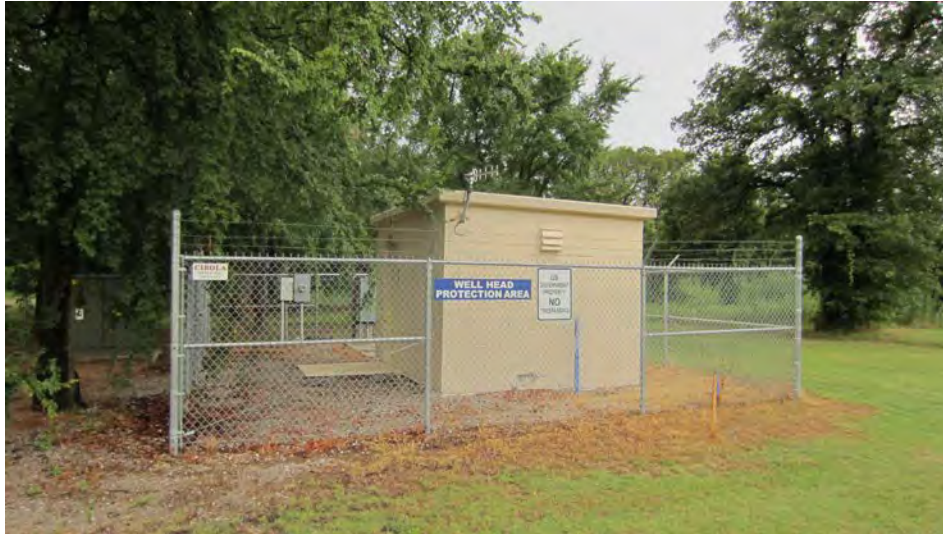
Typical wellhead enclosure at the Winstar World Casino and Resort.
